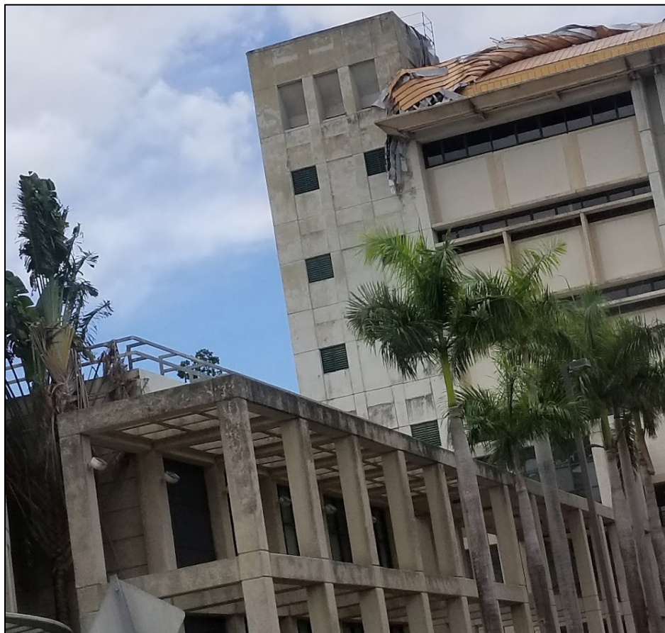
Figure 4-4: Damage to Commercial Structure Visible One Year After Hurricane Maria
