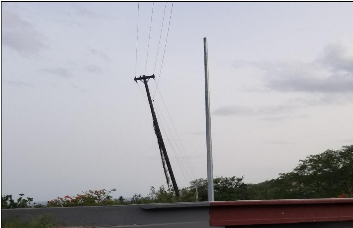
Figure 4-13: Damage to Electrical Grid
