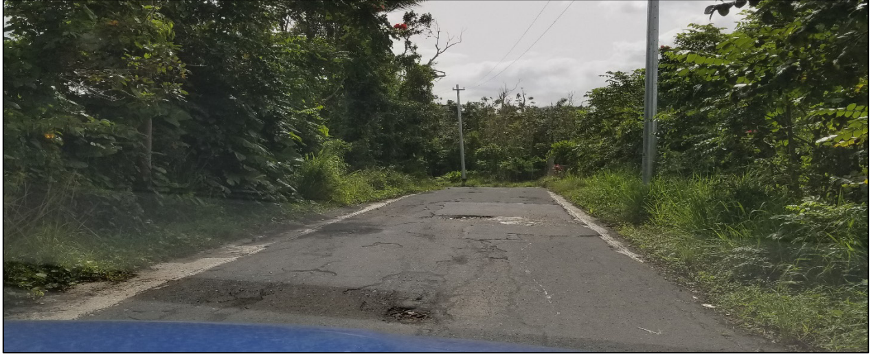
Figure 4-9: Rural Road Damage
