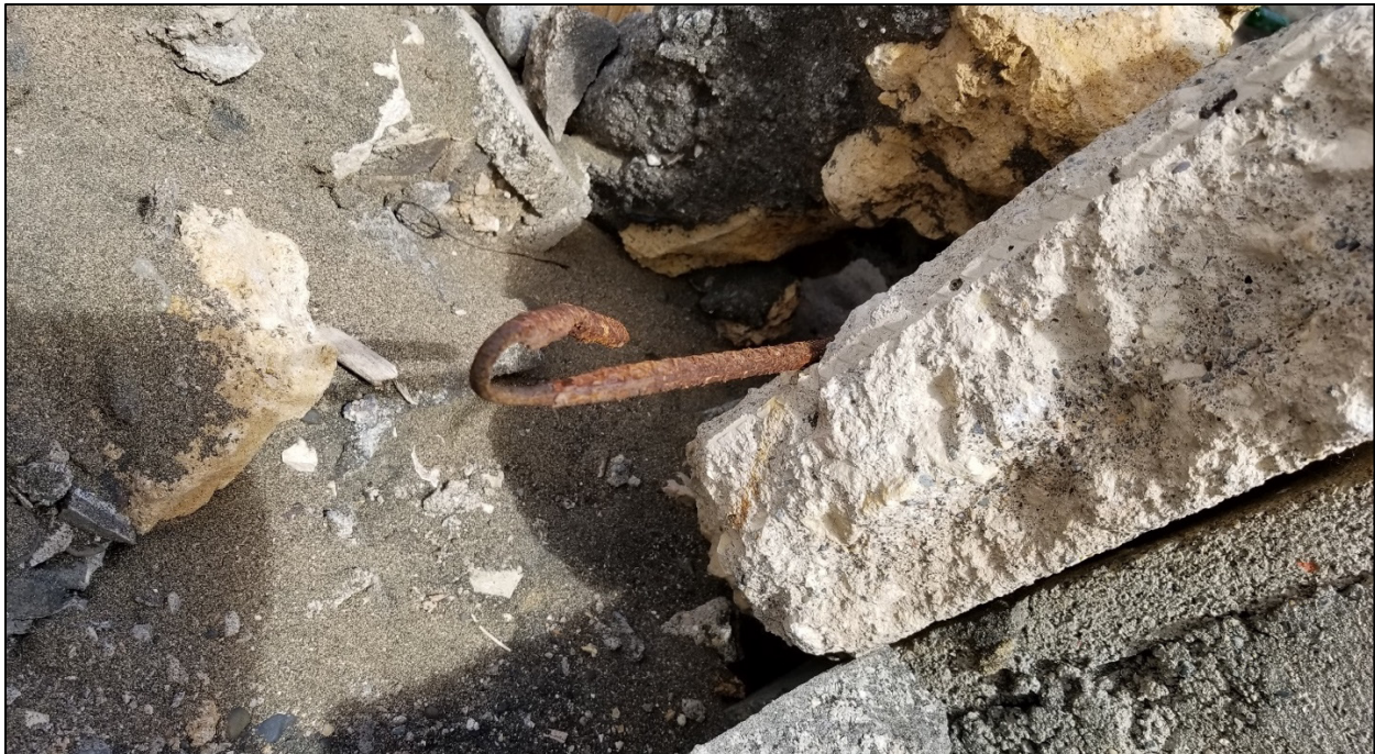
Figure 4-5: Results of Delaminated Rebar Exposed to Elements
